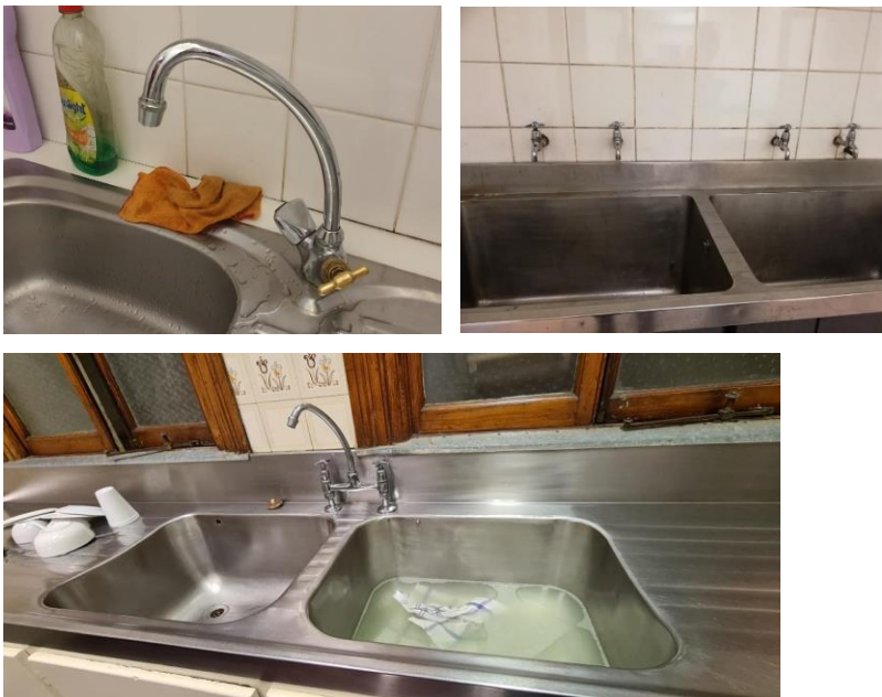
Figure 21: Kitchen tap fittings.
