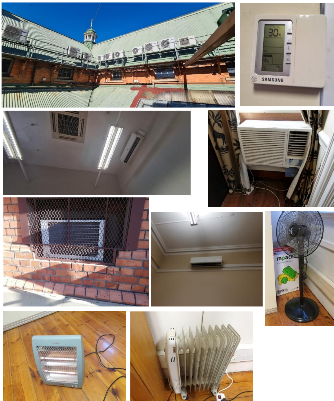
Figure 9: A collection of the split units (wall, through-wall and ceiling cassettes) and personal heating and cooling appliances observed throughout the building.
