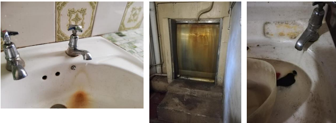
Figure 20: Leaking taps and fittings shown to be a long-term problem, as illustrated by stains in the basins and urinal in the basement.
