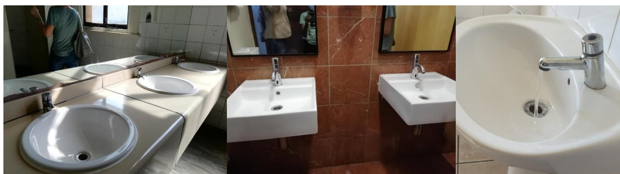
Figure 18: Examples of the various tap fittings and showing the high flow rate of the push taps.
